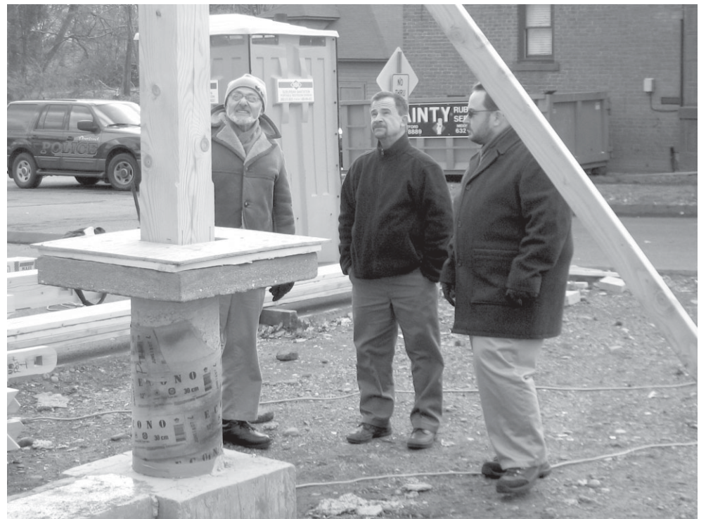
Howard Rosenbaum, Rick Kelsey and Jim Tripp admire construction at the site of the new Brownstone Arch Pavilion on Tuesday.
