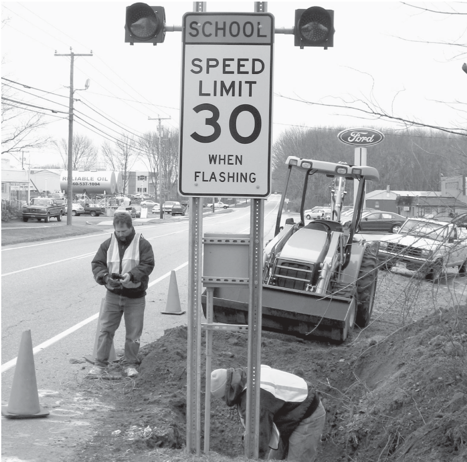
Installation of new signs and timed flashing lights in school zones along Colchester's Norwich Avenue is intended to make that busy thoroughfare safer for school children.
