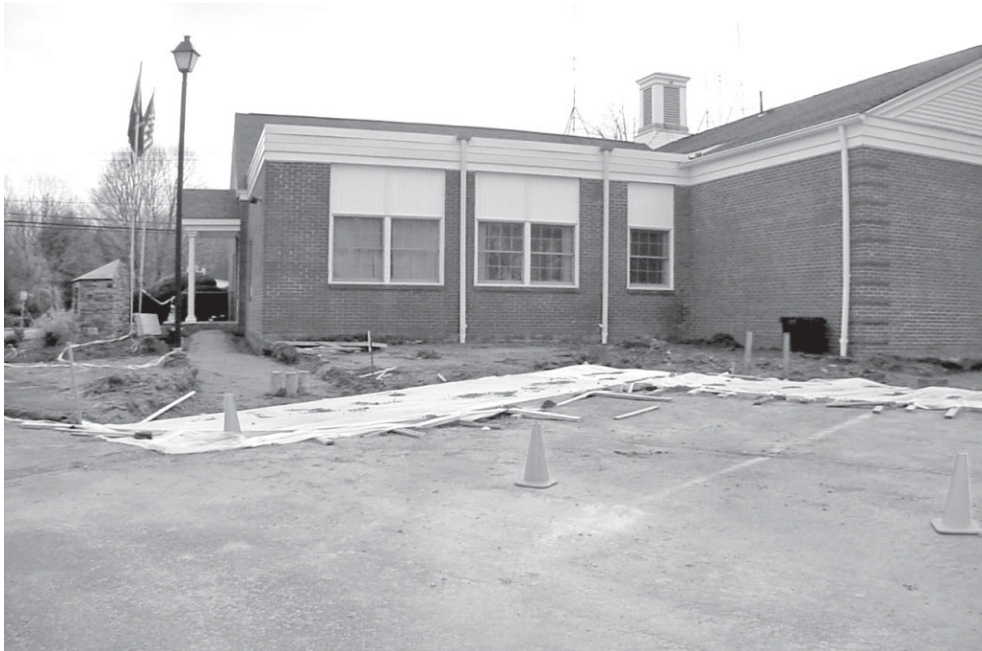
Work is underway at Town Hall to make the building ADA compliant. The structure was once an elementary school prior to construction of the current Elmer Thienes-Mary Hall School.
