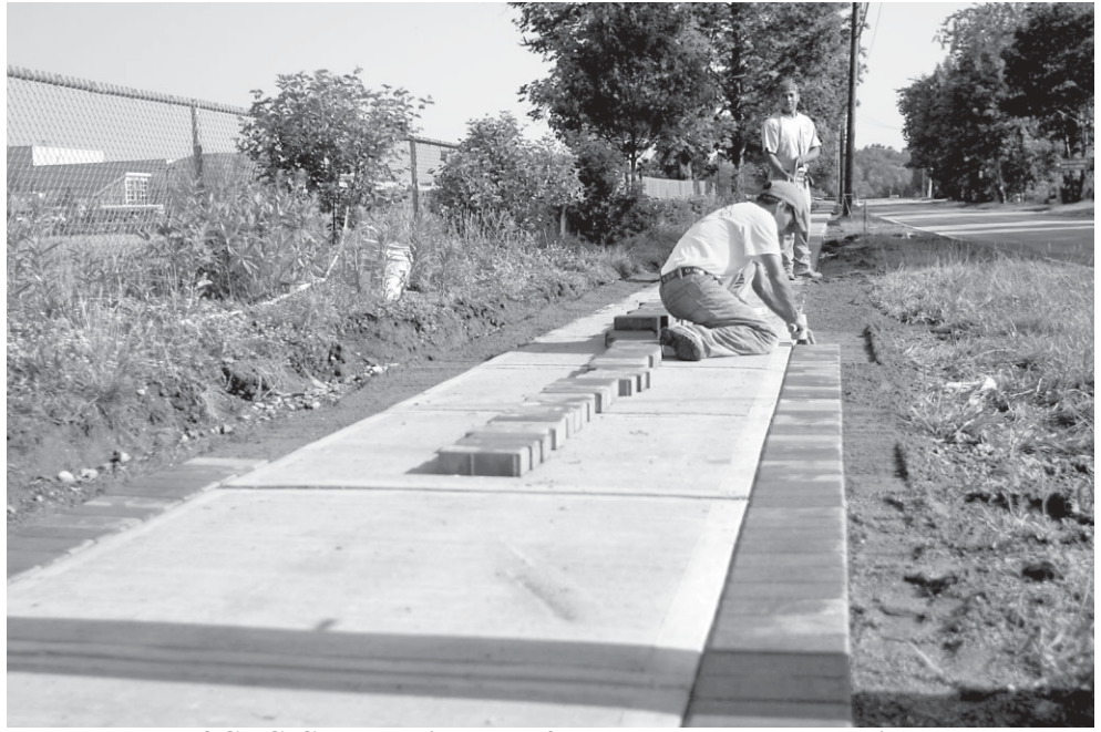
Employees of GEG Construction out of Massachusetts, work to install pavers on the sides of a new concrete sidewalk along Wall Street. Hebron is wrapping up work on the first phase of sidewalk installation in the center of town.
