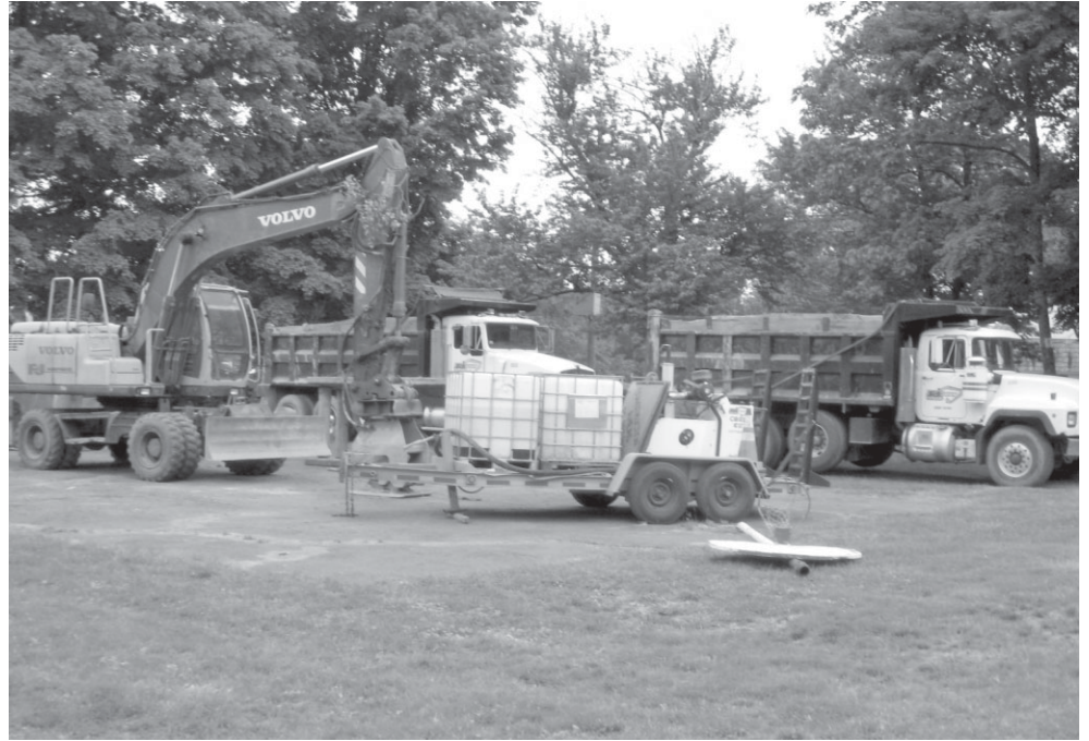
The town center and Lake Terramuggus sewer projects are finally underway. Shown here is construction equipment, after hours, in front of Town Hall.
