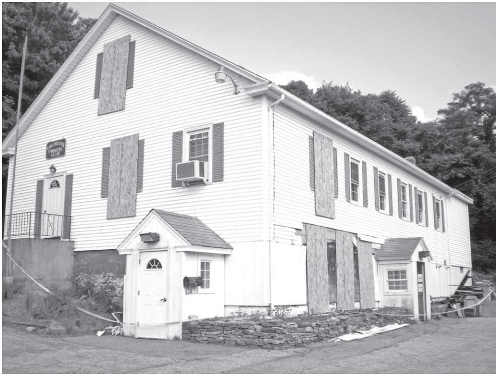
Significant damage was done to the Colchester Farmer's Club bar area after a fire broke out early Saturday morning.
