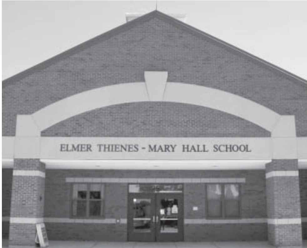
Mold was discovered under the stage in the community room at Elmer Thienes-Mary Hall Elementary School this August. On Tuesday, selectmen appropriated $3,200 for abatement and a topical treatment of the mold.
