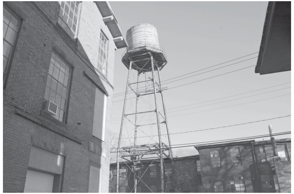
A dilapidated water tower, located at the corner of Summit and Watrous streets, has begun to tilt in recent months, drawing concern from town officials who want the structure torn down.
