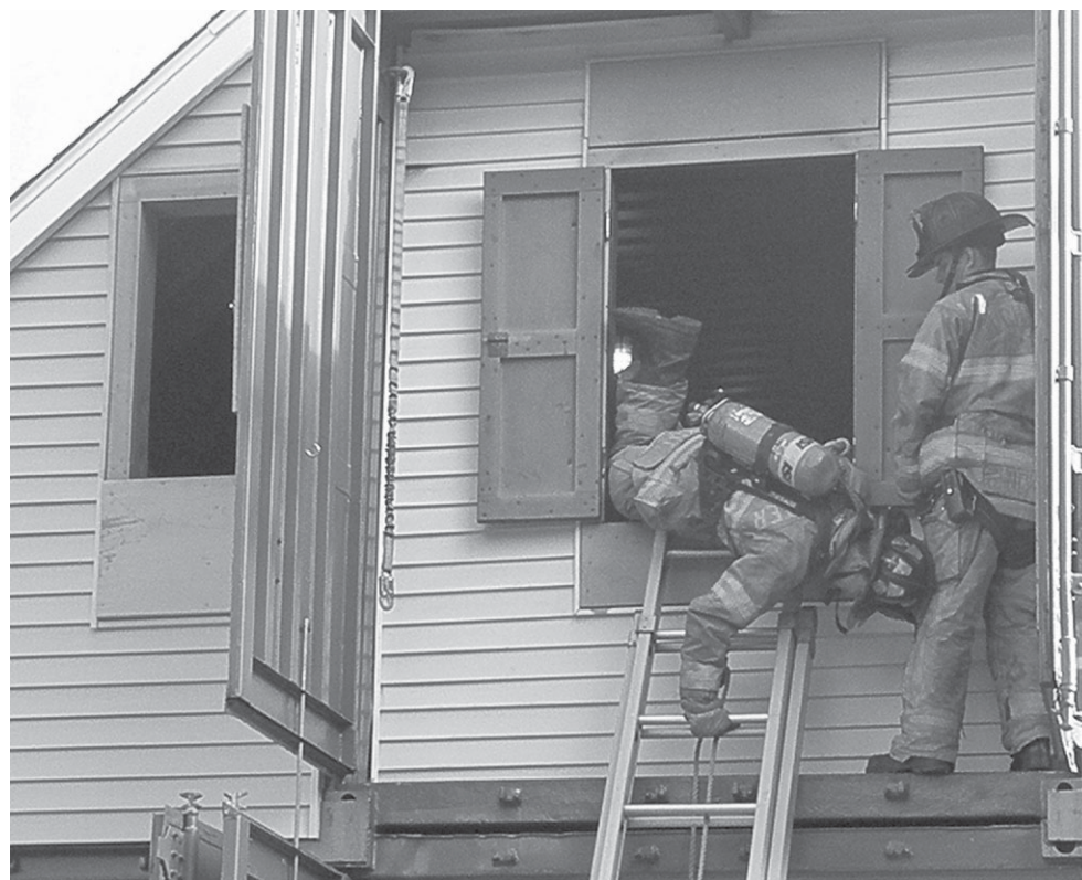
Firefighter Tony Skut demonstrates the way firefighters have to exit burning buildings at the new "burn house" in Colchester, with volunteer firefighter Keith Erickson nearby for safety.
