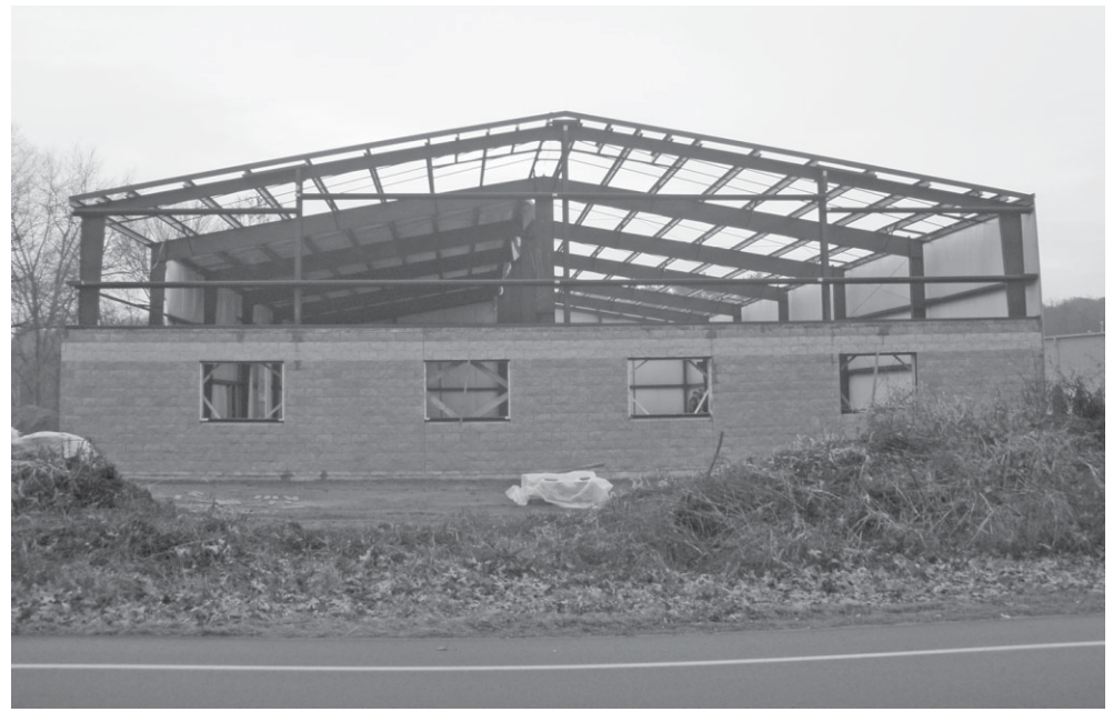
The future home of Marlborough Plastics, located at 350 North Main St., is eight weeks into construction. Photo by Bailey Seddon.
