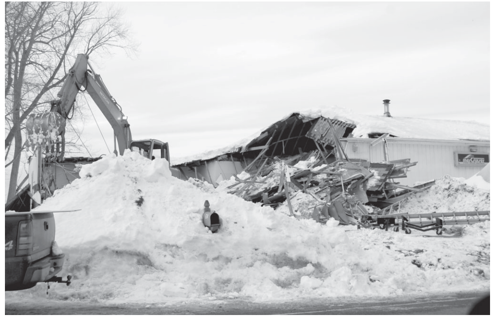
Four buildings collapsed in Portland last Thursday, Jan. 27, including Middlesex Marine, pictured above. Town officials said the large glass window in the showroom buckled under the weight of the snow.
