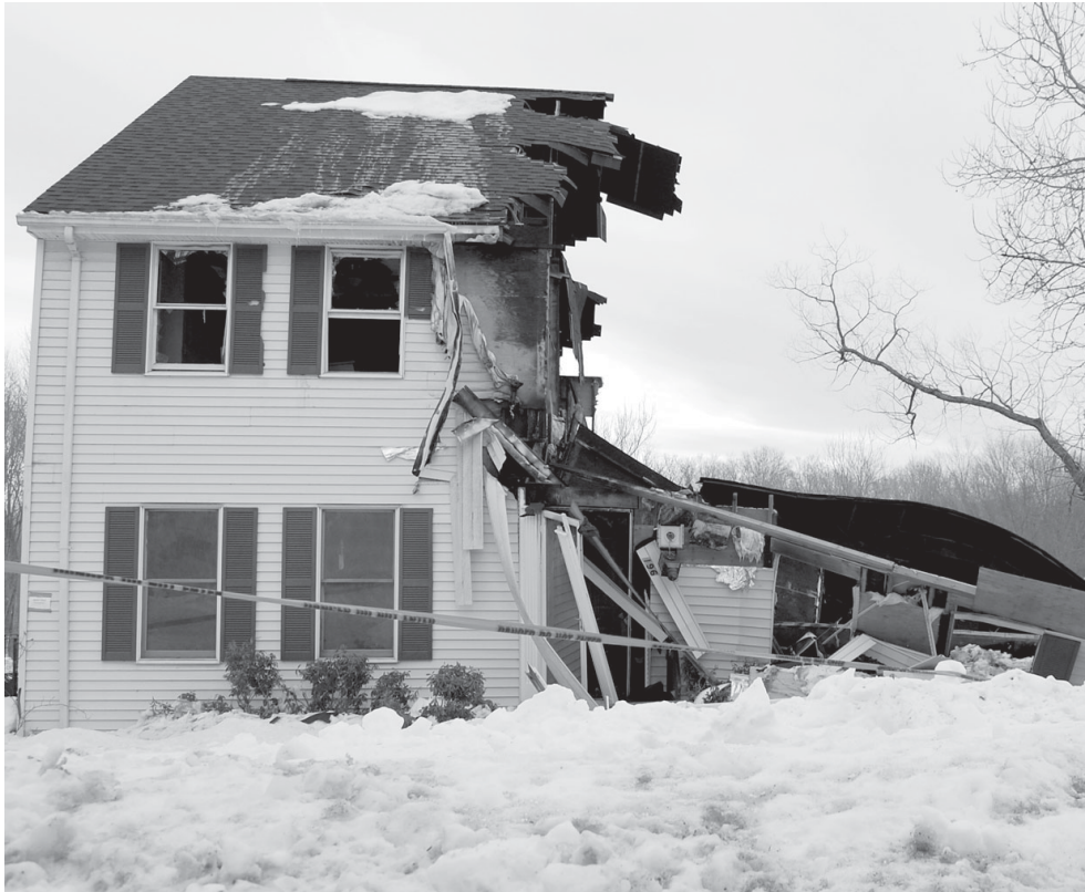
A propane leak in Portland last Saturday led to an explosion, destroying a Summer Street duplex and injuring two firefighters – one seriously. The leak was caused after a backhoe hit the valve of an underground propane tank, fire officials said.
