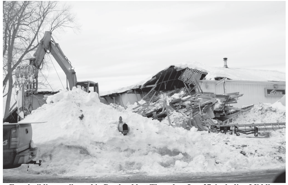
Four buildings collapsed in Portland last Thursday, Jan. 27, including Middlesex Marine, pictured above. Town officials said the large glass window in the showroom buckled under the weight of the snow.
