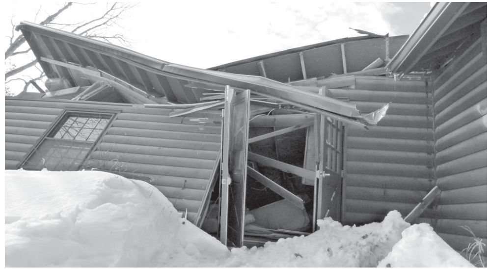
Selectmen denied a request from the 4-H Camp to waive its building fees to reconstruct Baldwin Hall. Pictured above is the building after it collapsed early February due to snow that had accumulated on the roof. Photo by Katie Tarka.
