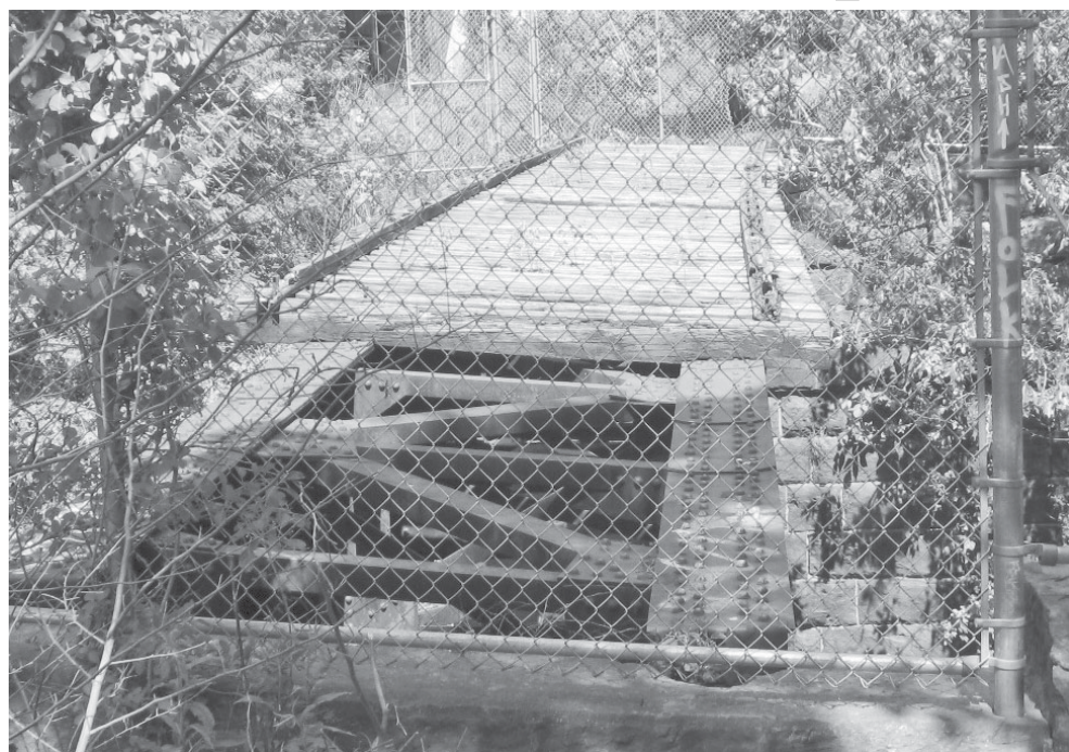
Construction is expected to begin this fall on an undeveloped portion of the Air Line Trail, extending the path into the Village Center. The plan involves upgrading the railroad bridge seen here, which people would be able to walk across to access either Watrous Street or a municipal parking lot, depending on which direction they're walking.
