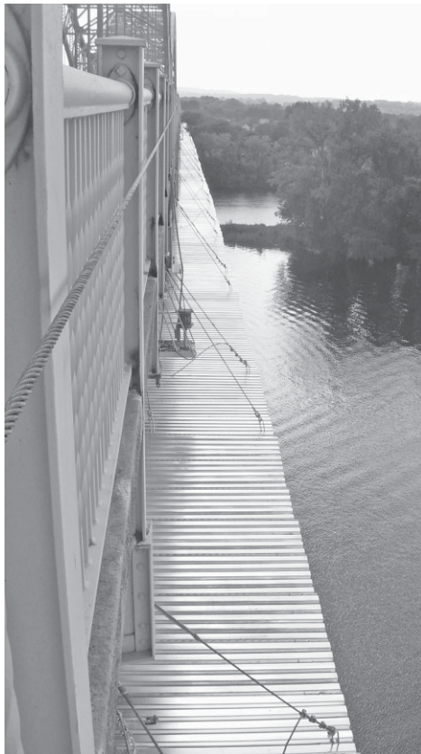
Shown here is the platform which the DOT and The Middlesex Corp. are utilizing as they complete work on the Arrigoni Bridge.
