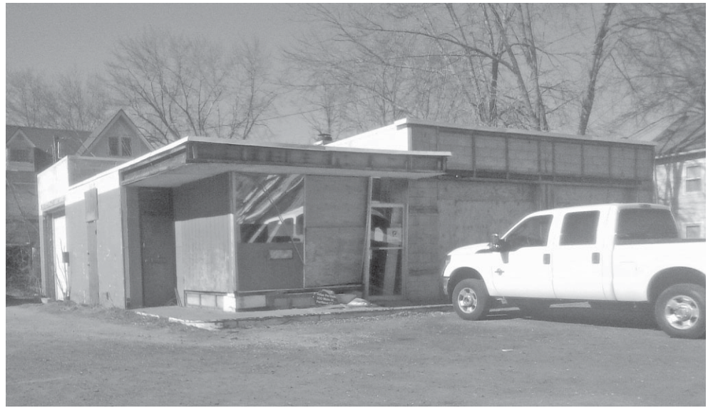
The former Mobil gas station on Main Street has been closed for well over a decade and has fallen into disrepair, causing many residents to call for its demolition. This week, the town was in discussions with the property owner to do just that.
