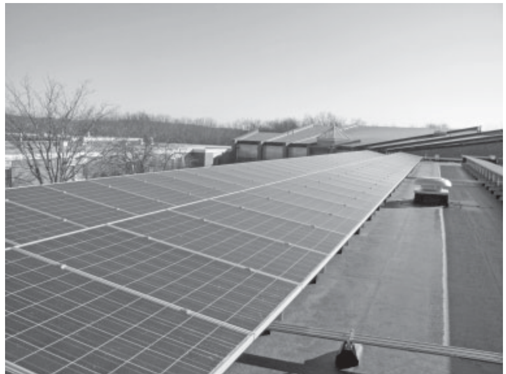
Now that a system of 442 Solar Photovoltaic panels are up and running on the roof of Gilead Hill School, sunshine equals savings. The school is expected to reap about $10,000 in electricity savings as a result of the panels.
