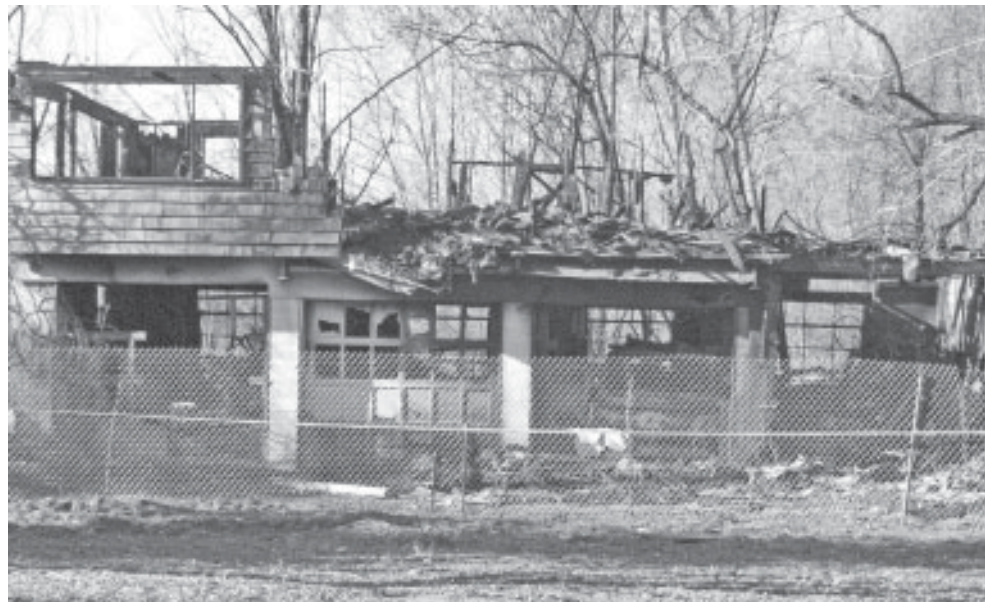
Pictured here is the aftermath of a reported explosion and structure fire to the residency at 474 Glastonbury Tpke. The abandoned four-car detached garage was engulfed in flames last Friday, Nov. 22, by an unknown origin.
