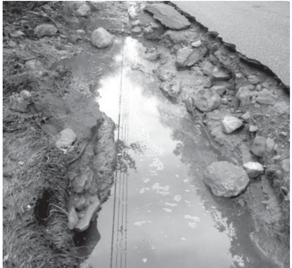
The aftermath of the dam break in Hebron left Jones Street with approximately 300 yards of dirt and rock flushed from the road. The road was closed early Monday morning and reopened later that day after additional gravel was replaced.
