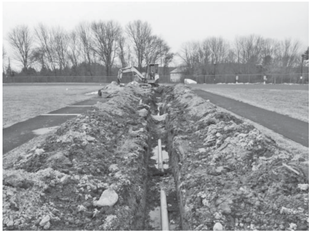
At Monday’s Board of Education meeting, recognition was given to individuals who volunteered during clean-up and repair efforts on school grounds last year. One of those recognized was Brien Belavander of B & J Construction Company, who installed a new drainage system for the long jump pit.
