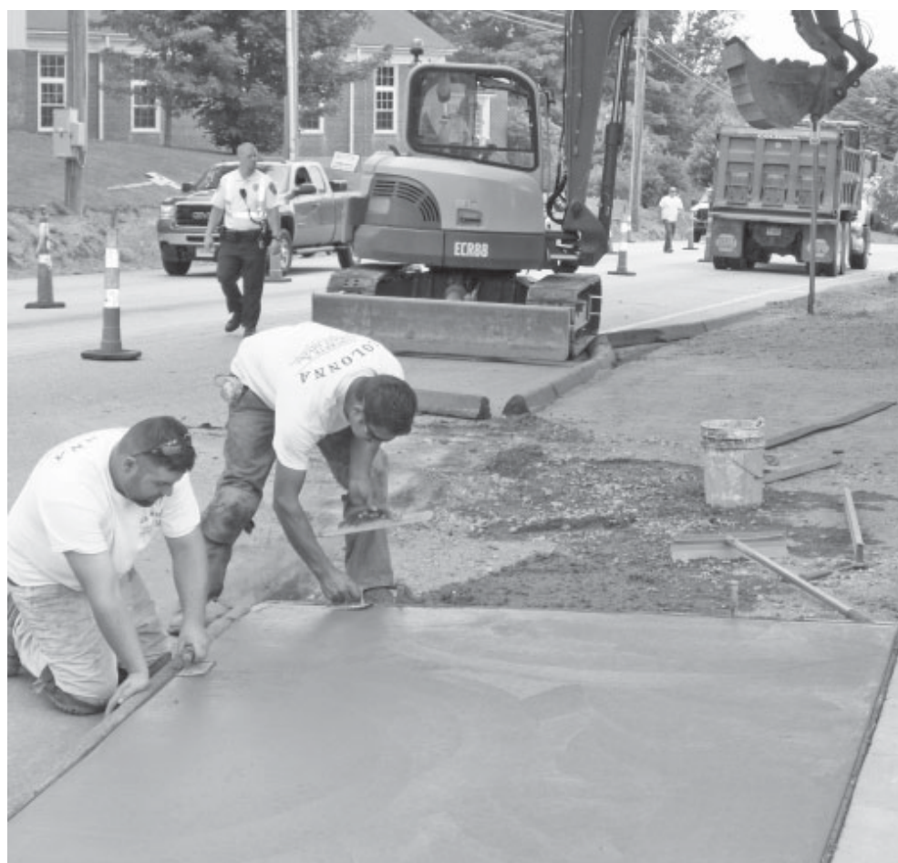
Construction workers lay down new stamp concrete on Linwood Avenue earlier this week, as part of the “Linwood Avenue Streetscape Project.”
