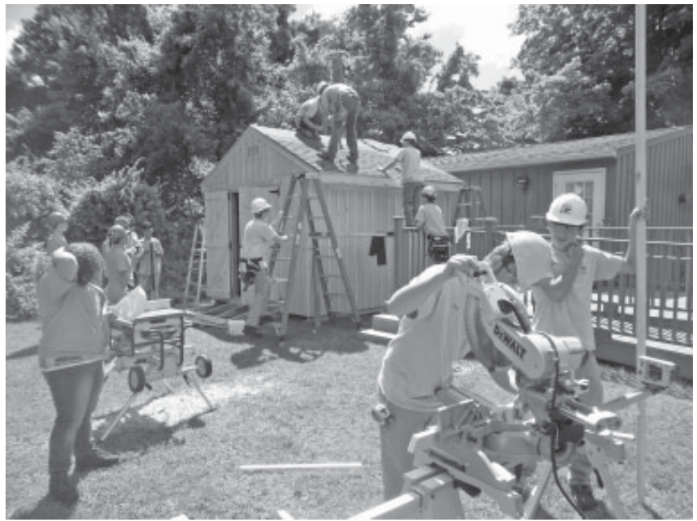
The Chatham Historical Society has a new, custom-made storage shed. The shed, at 10'x12', will store the society's signs. Students from Vinal Technical High School built the shed as a community service project.
