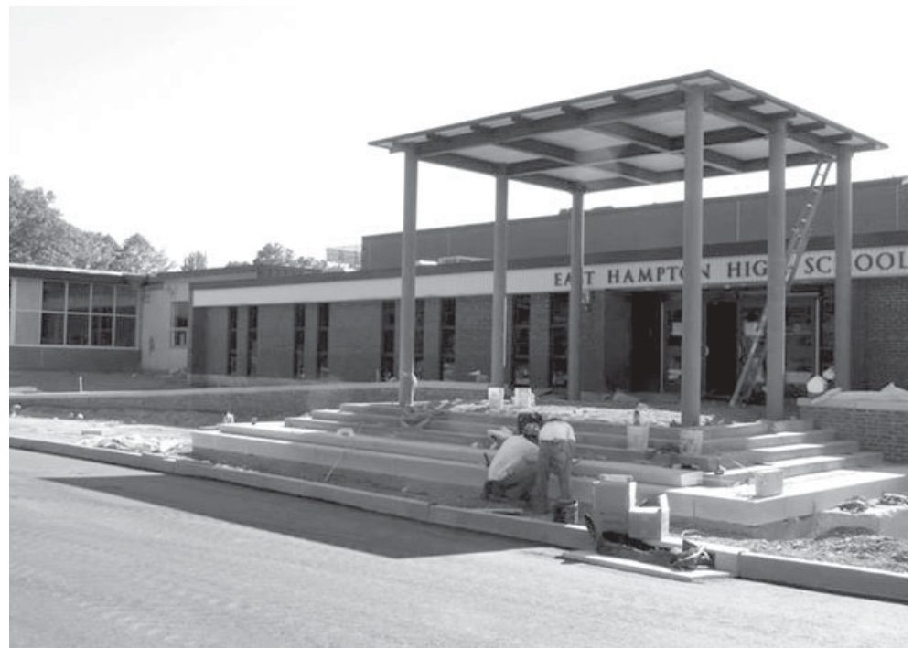
A covered entryway to East Hampton High School's main entrance is just one of several new features added to the building over the summer, along with a new front parking lot, an expansion to the cafeteria, a remodeled gymnasium, a new science wing and much more. Photo by Cynthia Abraham.
