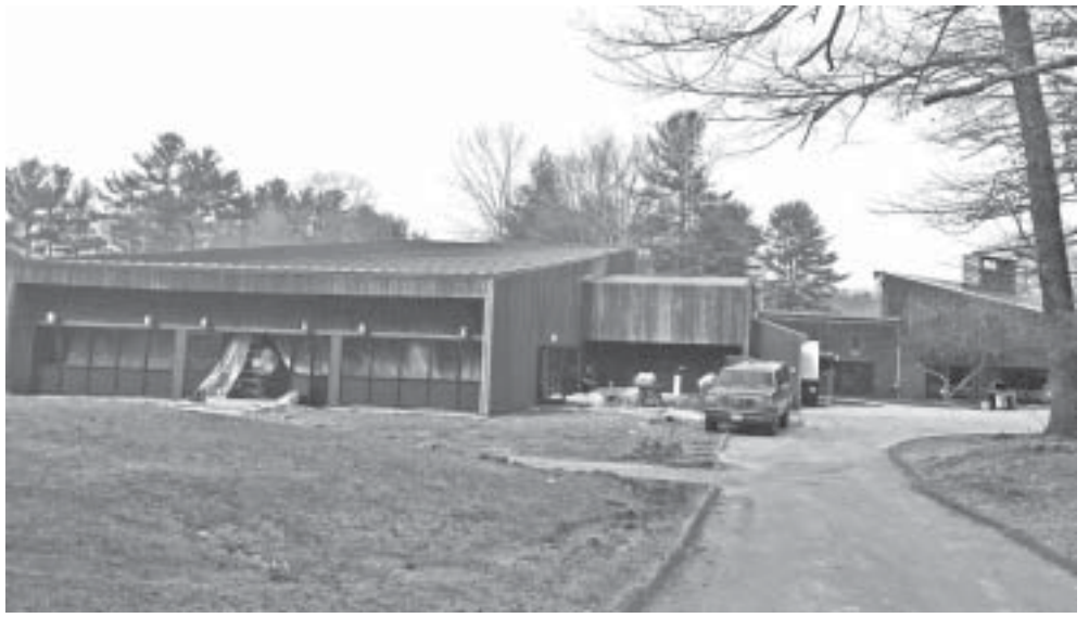
Work on the outside of the main building at The Hemlocks Center includes the replacement of siding and some of the windows. Intern Kerry Kincy is also hoping to gather a group of volunteers to help on the grounds, cleaning the nature trails and painting swing sets among other things.
