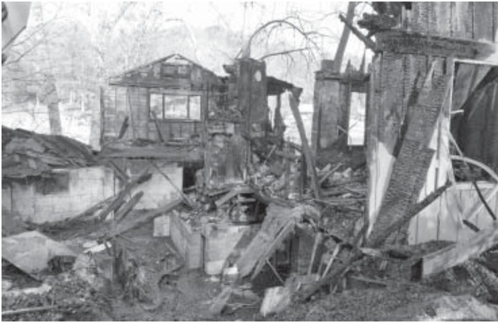
A former Murphy Road residence is left in utter devastation following a house fire last Thursday, Nov. 9.
