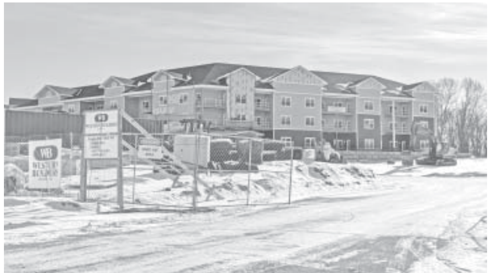
Construction at Colebrook Village is entering the home stretch. The assisted living community is slated for a May opening.
