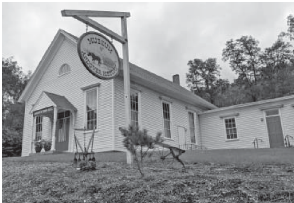
The Museum of Andover History, which is housed in the Old Town Hall, has a leaking roof and the town is looking to fix it.
