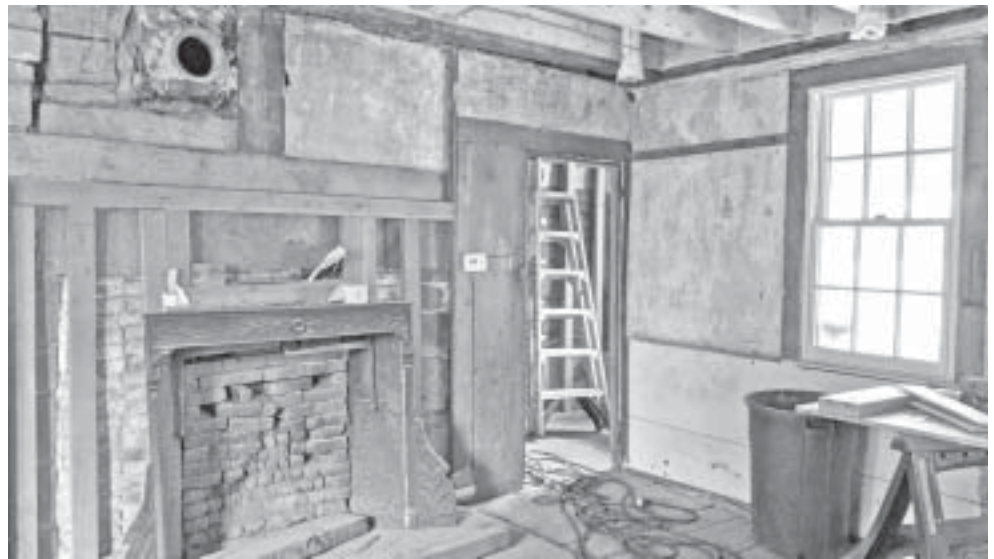
The L-wing of the Peters House is being restored as a museum. Seen here is the metal framed mantel on one side of the dual fireplace, the other side has a distinctly different brick and rubble mantel.
