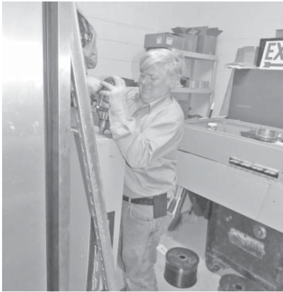
Hard at Work... Hebron resident Dan Larson does some electrical work during the renovations of Phelps Hall at St. Peter's Episcopal Church. The renovation project is moving more quickly than expected. See related story on page 18.
