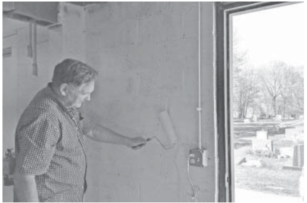
Ron Churney paints a wall during Phase 2 of renovations of Phelps Hall at St. Peter's Episcopal Church.
