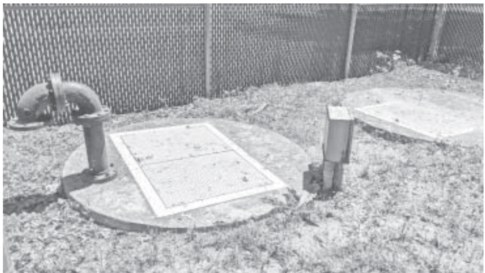
Pictured here is a pump station in Amston on Route 85. The town is considering updating all nine pump stations in town as they are reaching the end of their useful lives.
