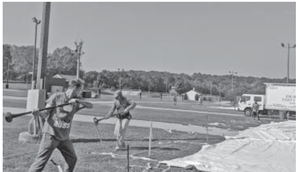
Workers from Durants Party Rentals in Danbury hammer supports in the ground for a tent for the upcoming Hebron Harvest Fair, which takes place Sept. 6 through 9.
