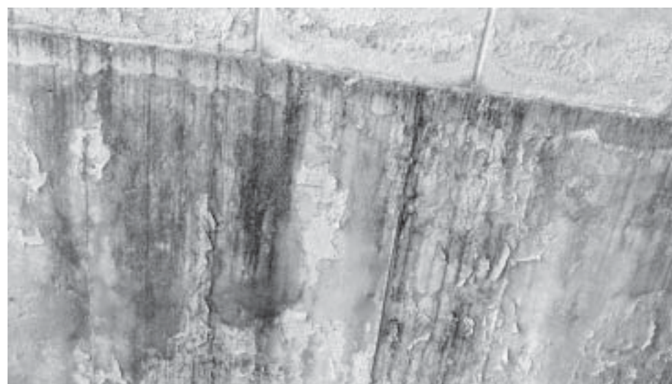
Mold stains appear in patches along walls and on the ceiling throughout the basement/garage of the Old Firehouse, which serves as the town’s senior center.
