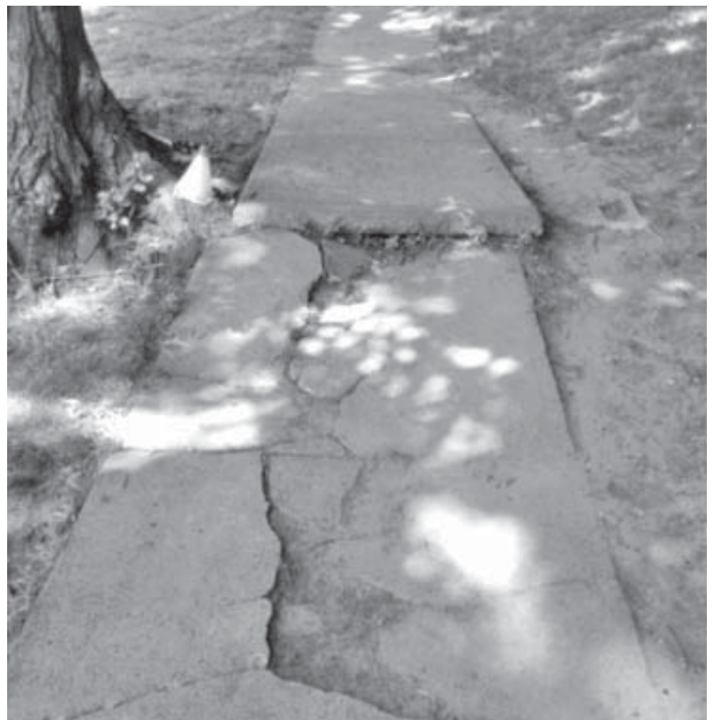
Deteriorating Main Street sidewalks, like this one at the intersection of Fairview Street, will be replaced now that the town has received a $204,358 grant through the state Community Connectivity Program.
