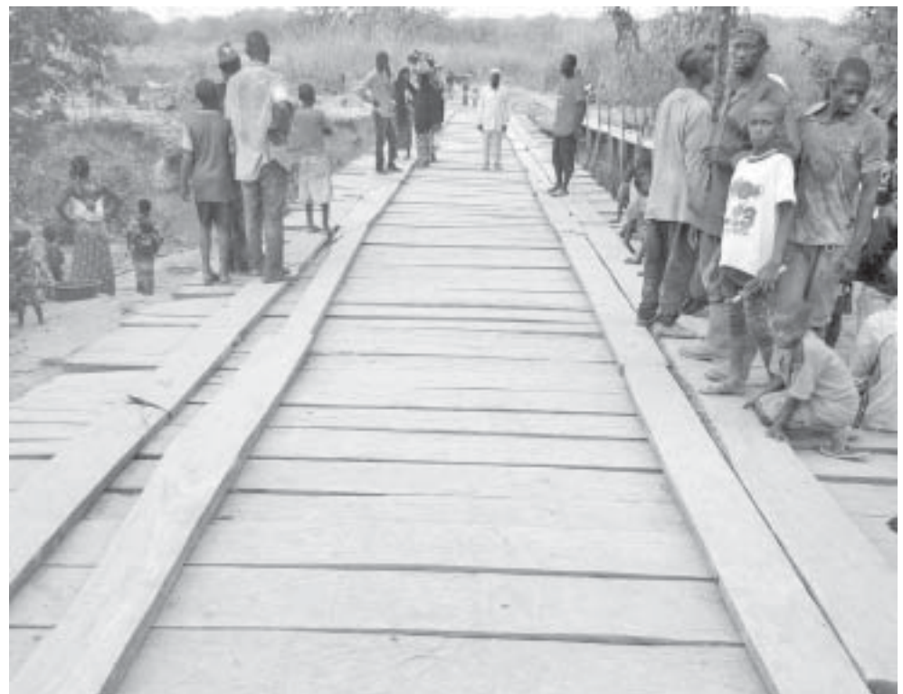
This bridge between the villages of Morowaya and Duako in Guinea, West Africa was sponsored by the Bolokada and Friends Village Project, which was founded by Hebron's own Carla Pomproicz. The next project on the list for the non-profit is to build a hospital in Morowaya.
