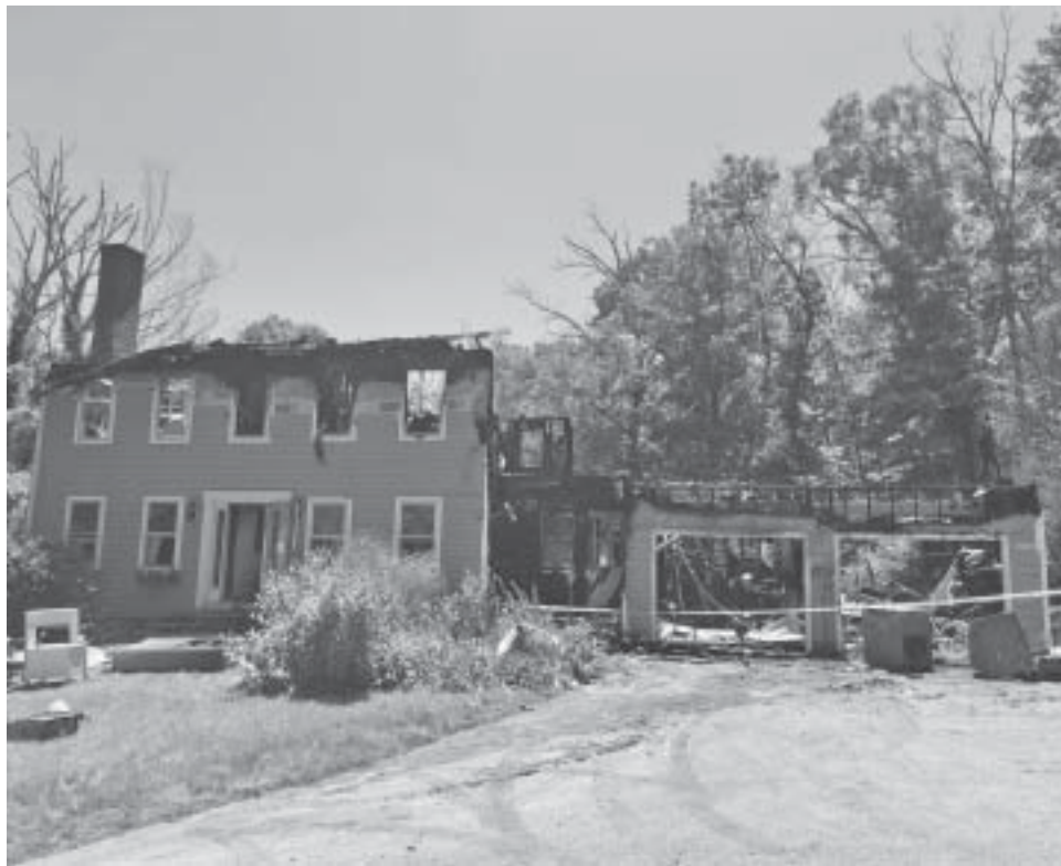
House Destroyed... This is all that remains of a Hebron home after fire ripped through it last Saturday afternoon. Nobody was home at the time of the blaze – but two dogs were rescued by a brave passerby. See story on page 10.
